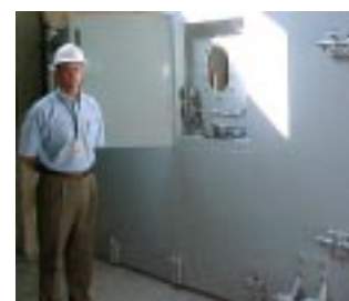
Hyde Griffith, Facilities Operations, shows off the first flood door.
